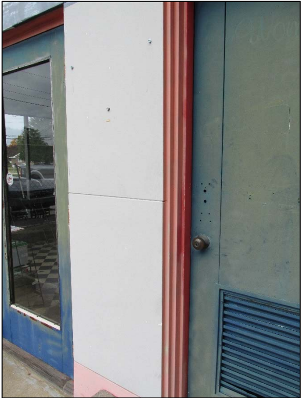
Figure 48. Exterior wall material, with added office door to the left and restroom door to the right.
